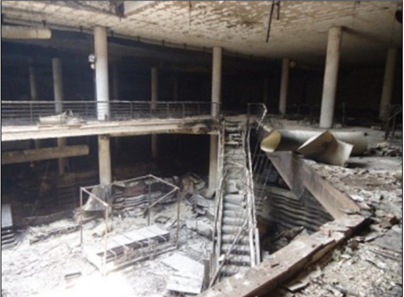
View of the inside of the Nakumatt Super Market after the fire and roof collapse.
