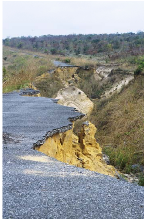
The road between Brazzaville and Mayama has not been maintained and is not passable in many places.
