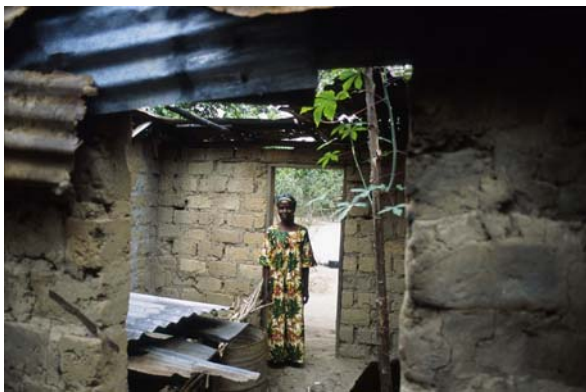
Mayama: A villager in her house destroyed during fighting in April 2002. Materials for reconstruction are always lacking.
