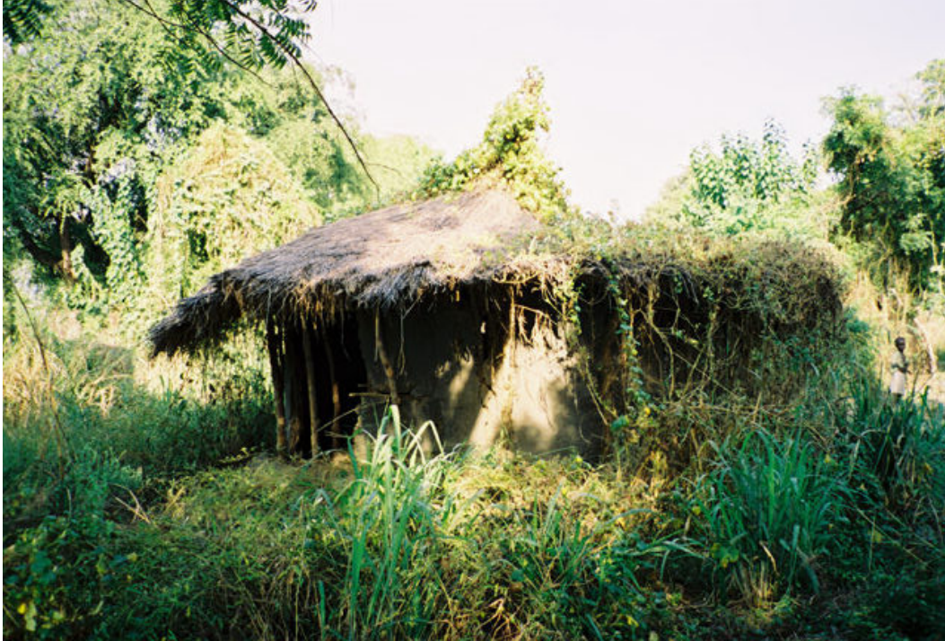
This house in Gambella town's Omminingah neighborhood was rebuilt by soldiers and highlander townspeople after they razed the neighborhood during the December 2003 massacre. The house was so poorly constructed that no family was willing to live in it, and its roof quickly collapsed. Similar houses are scattered throughout Gambella town. © 2004 Human Rights Watch
