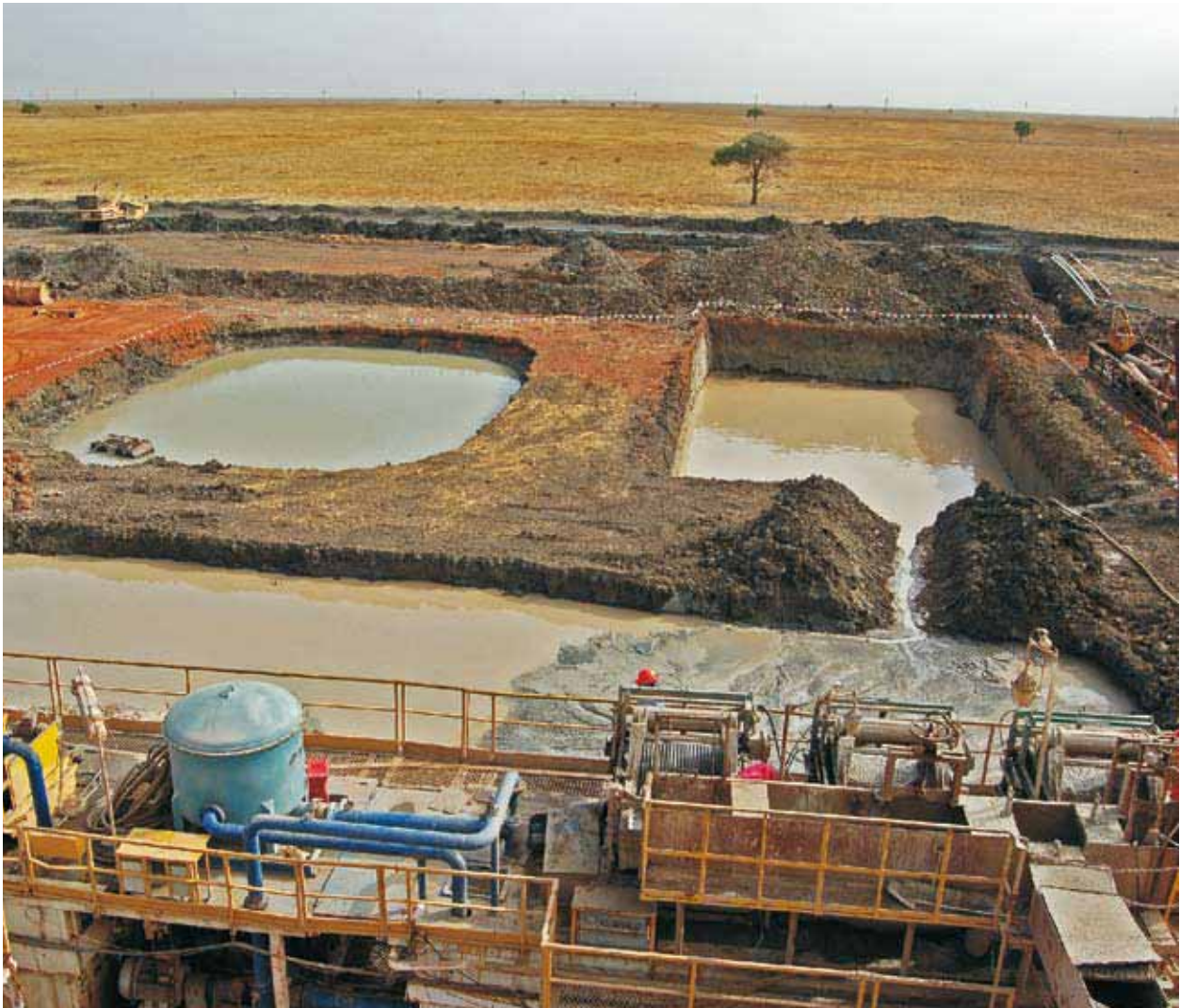
Oil well drilling pits such as these at Heglig are normally remediated after use. At present, however, there is no oversight of the oil industry's performance or detailed environmental standards for such work
