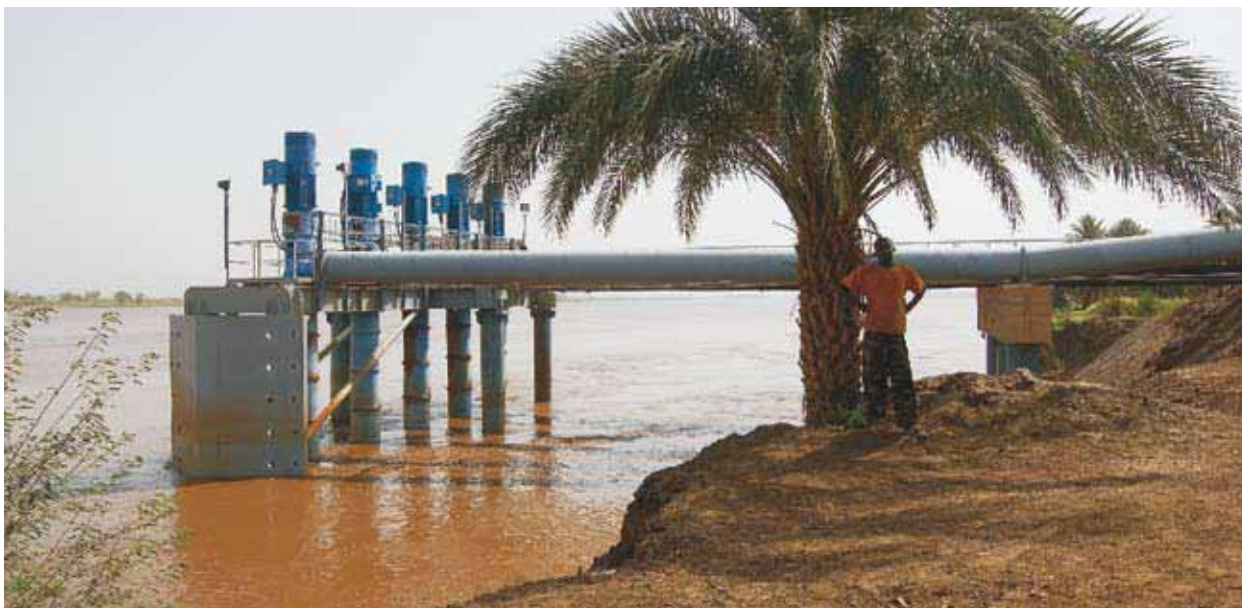
Riverbank erosion removed the supports of this irrigation pump intake system within months of its installation, and threatens to destroy it completely. Without mitigatory measures, the site is not suitable for such a project
