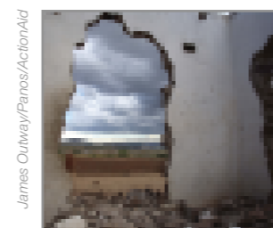
A demolished house near Ga-Puka.
