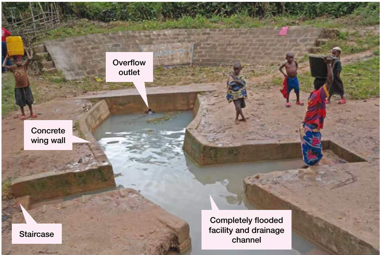
Constructed in July 2006, the Vala spring box in Libenge, Equateur Province, fell into disrepair by 2008, forcing local communities to tap seepage around the spring box or travel longer distances in search for water
