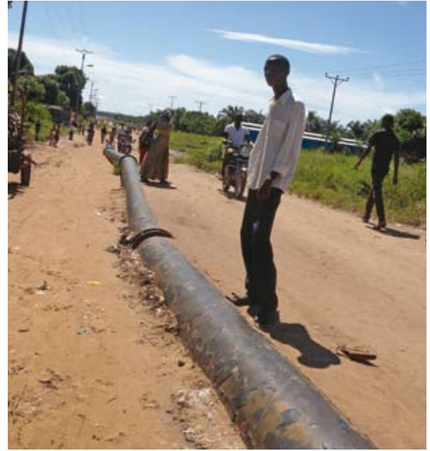
REGIDESO's main transmission pipeline in Mbuji-Mayi is exposed to a high risk of structural deterioration. This occurred in February 2010 when a catastrophic failure caused the sudden loss of millions of liters of water and damage to surrounding property. Water delivery was cut-off for several weeks in this city of over one million residents (above and below)
