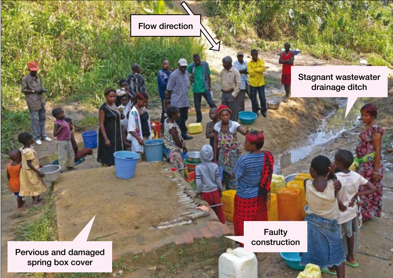
In Kalima, Mainema Province, the Baganda spring box combines several features of poor construction and maintenance including: reduced flow rate, damaged spring box cover, sediment build-up and clogging of the drainage ditch, lack of fence enclosure and upslope footpaths increasing erosion and contamination risks
