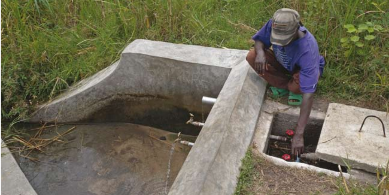
The Djokojo spring, which has now almost run dry, was originally developed to meet the water needs of displaced and local communities on the outskirts of Bunia, Ituri District
