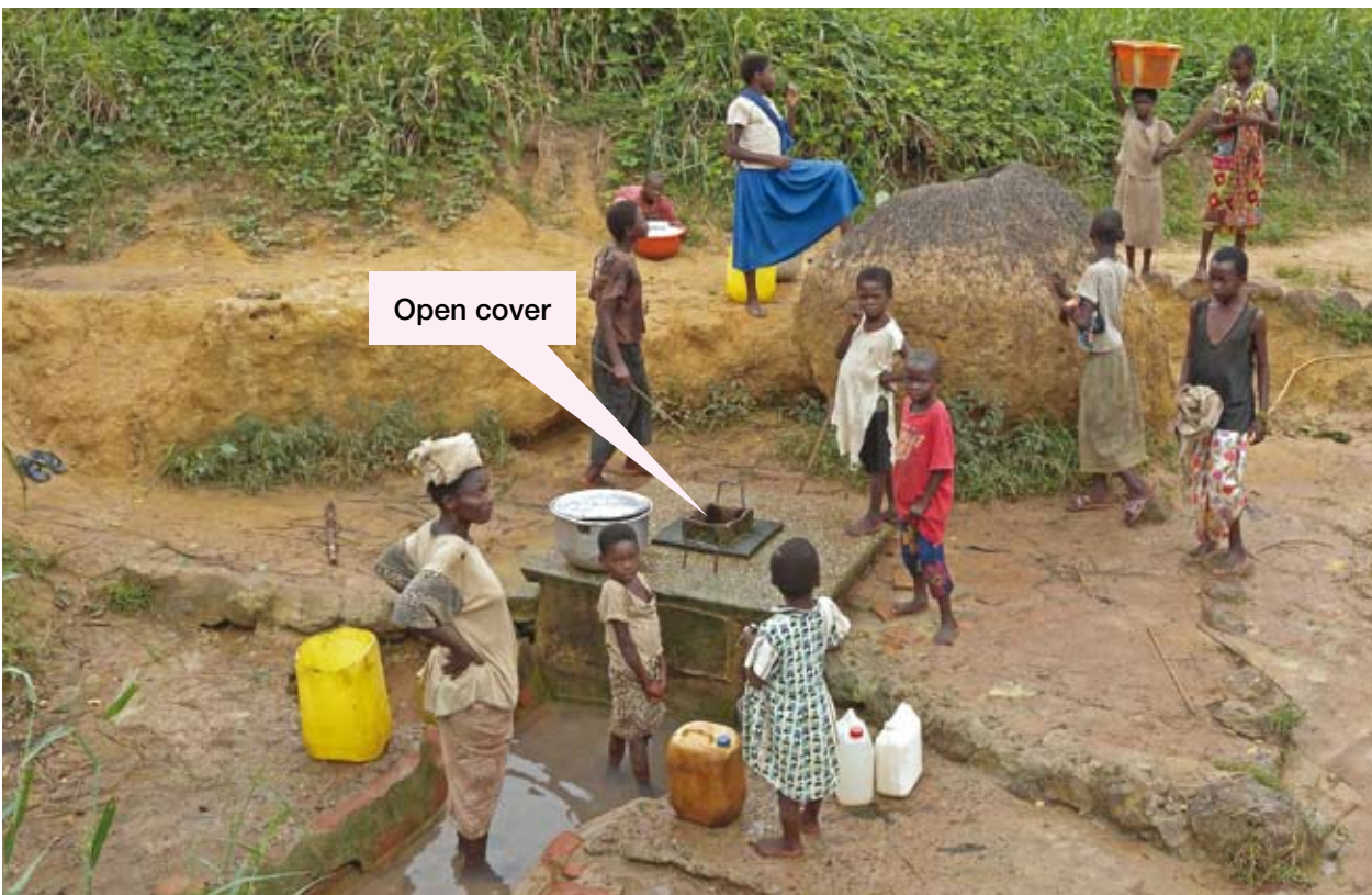
The protective cover of this spring box is partially exposed rendering contamination inevitable. Note also the lack of any diversion ditch and fence around the site to protect from pollution. (Denge spring, Libenge, Equateur Province)
