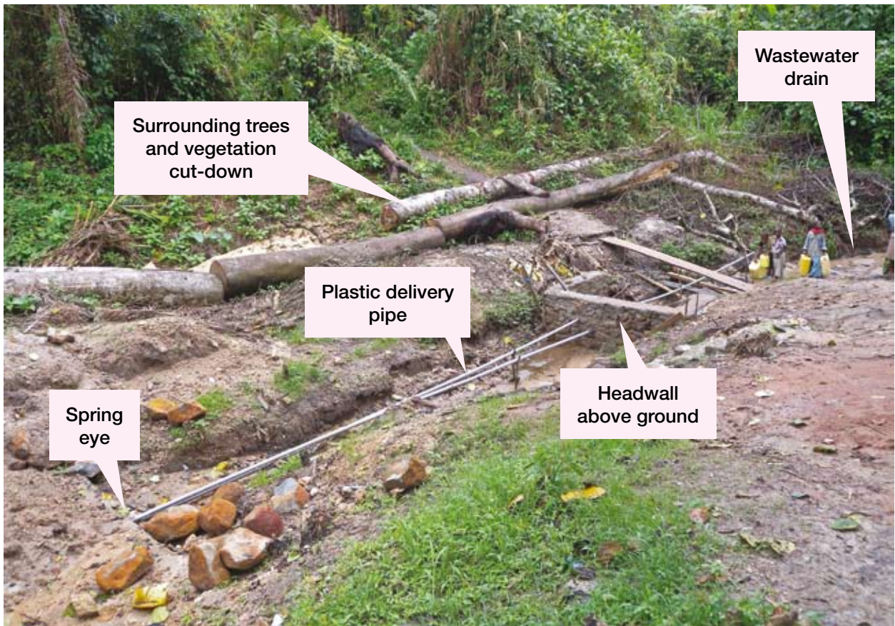
Work in progress: construction of a retaining headwall in the village of Kandate in Ituri District
