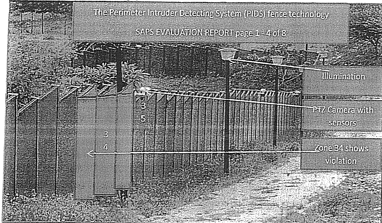
Figure 6: Perimeter Intruder Detecting System
